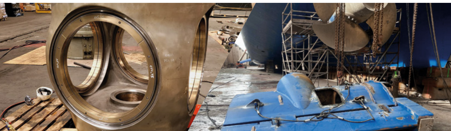
Repairs in Dry Dock – Rudder, steering gear, hub and Promas. Location: Marseilles, France.
